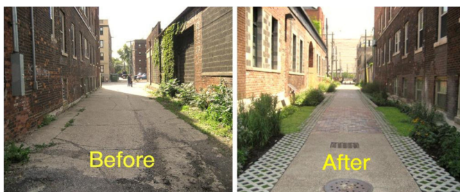
Cool Pavement, before and after a sustainable reconstruction Chicago's Green Alley Program
